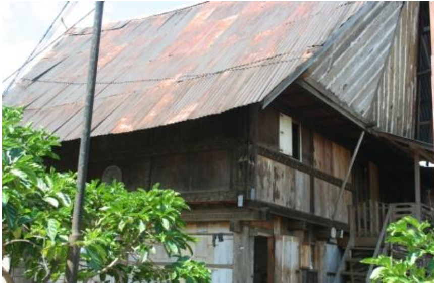
Image 8. One of the traditional architecture which isn't in a good care eventhough this heritage is under cultural preservation.
